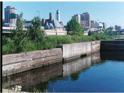
Stormwater pipe entering Slip 2 at the Bayfront Living Water Garden site.
